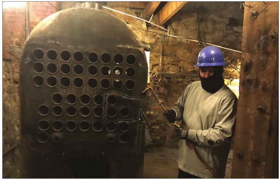
Contributed photo Horsley team member Eliazar Garza-Gutierrez begins cutting up the boiler with his blow torch.
